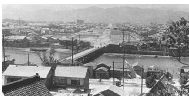
Photo 4-2 The 100-meter road under construction as seen from Hijiya Hill (May 12, 1952) (Collection of the Hiroshima Municipal Archives)
