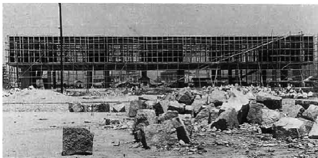
Photo 4-1 The display hall under construction (today’s Peace Memorial Museum Main Building) (Taken on July 1, 1952. Collection of the Hiroshima Municipal Archives)
