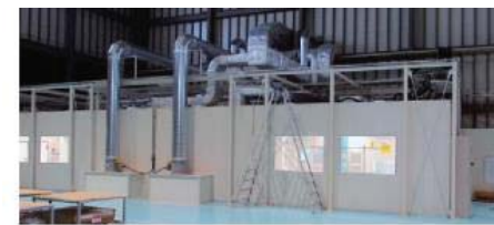
Large Clean Room
